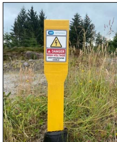
Figure 5 - ESB Marker Posts
