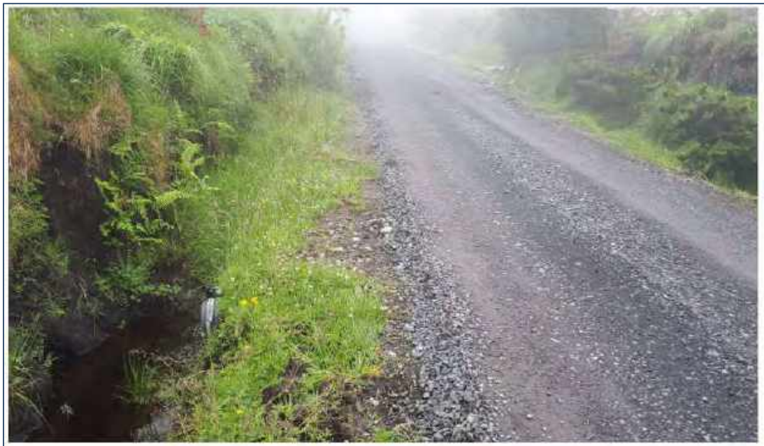
Photo 6: Crushed Aggregate Road, Pipe Culvert Across Road, and Drainage Ditches on Both Sides of Road
