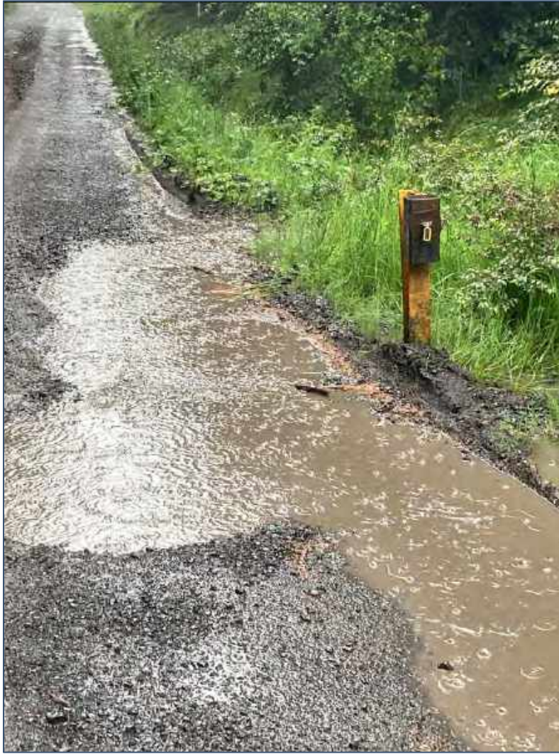
Photo 7: Suspended Sediments in Road Runoff Entering Drainage Ditch, 18 June 2023
